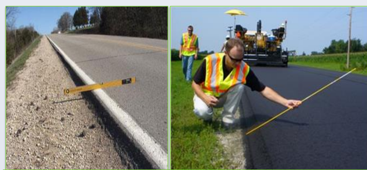
An Edge Drop-off. Hallmark et al. (2006) A typical Safety Edge. Source: FHWA.
